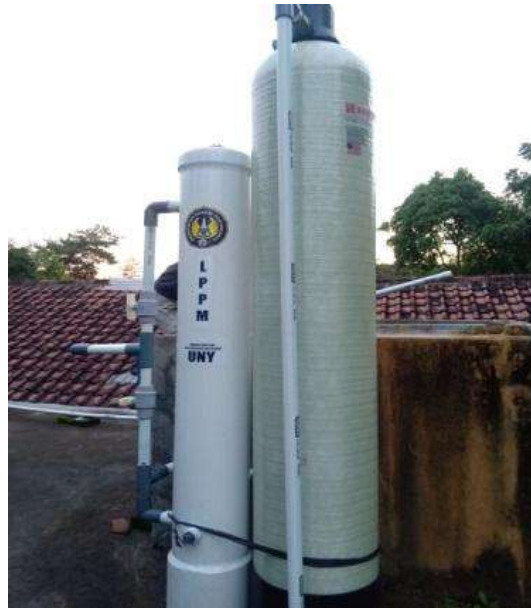
Figure 1. Series of Column Adsorption Method Water Treatment Equipment using Natural Zeolite Adsorbent and Activated Charcoal
