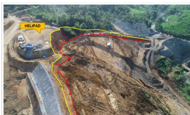
Figure 1. Documentation of landslides on the right side of the main dam abutment
