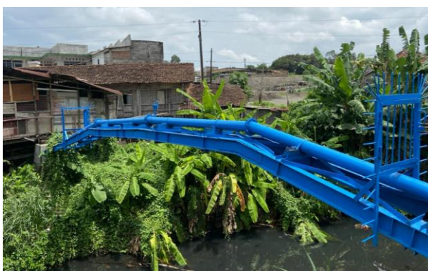
Figure 13. Location of the new pipe bridge next to the existing pipe bridge
