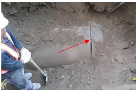
Figure 2. Sinkhole occurrences due to defective sewers [1]
