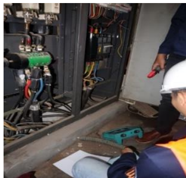
Fig. 7. Measurements on PT ABC's electrical panels
