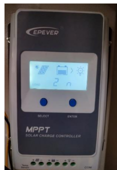
Fig. 10. Measurement via MPPT Epever Tracer screen monitoring
